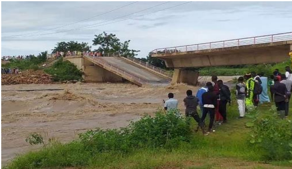
Photo 3: Destruction of the bridge linking the Far North region to the rest of the country following heavy rainfall. Source: Château news.com (August 2020)
