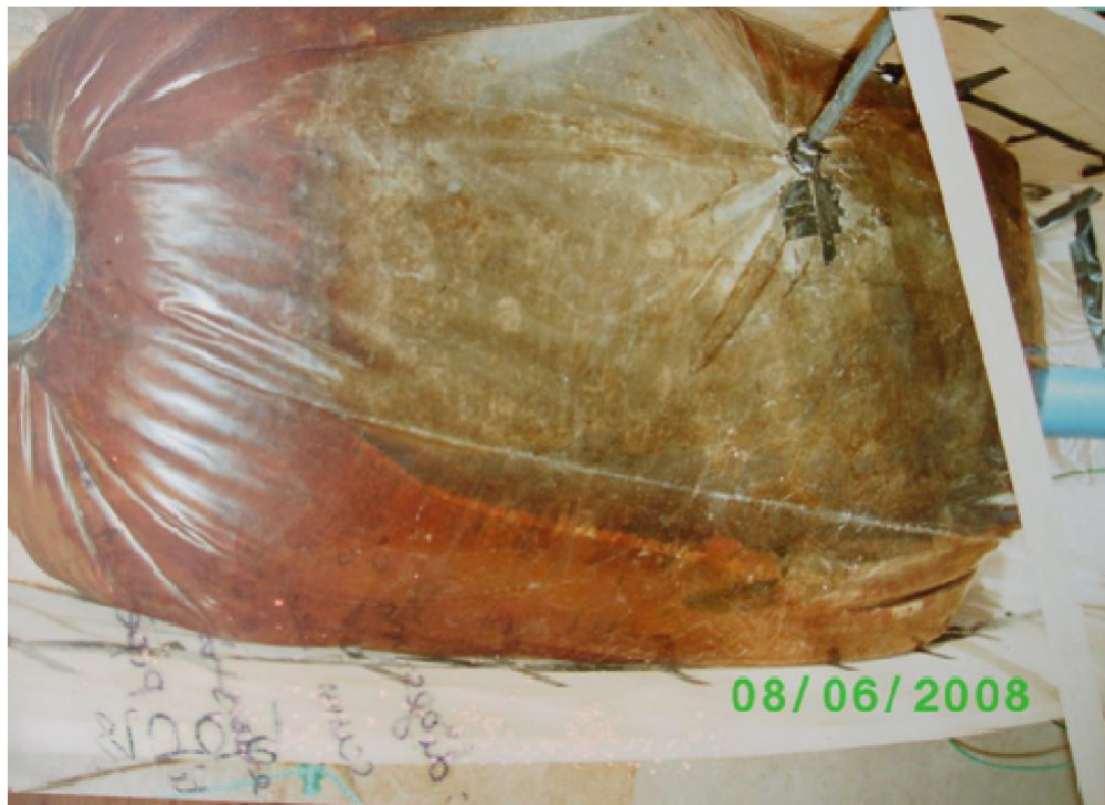
Figure 6. The anaerobic digester.
